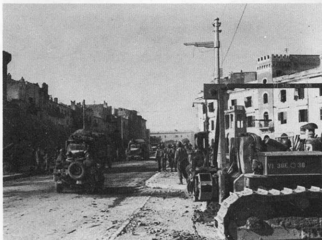
Men of the 1st Battalion of the 36th Engineers were on hand to bulldoze the wreckage aside and they soon had the traffic moving again. Although inexperienced to the rôle, three days
