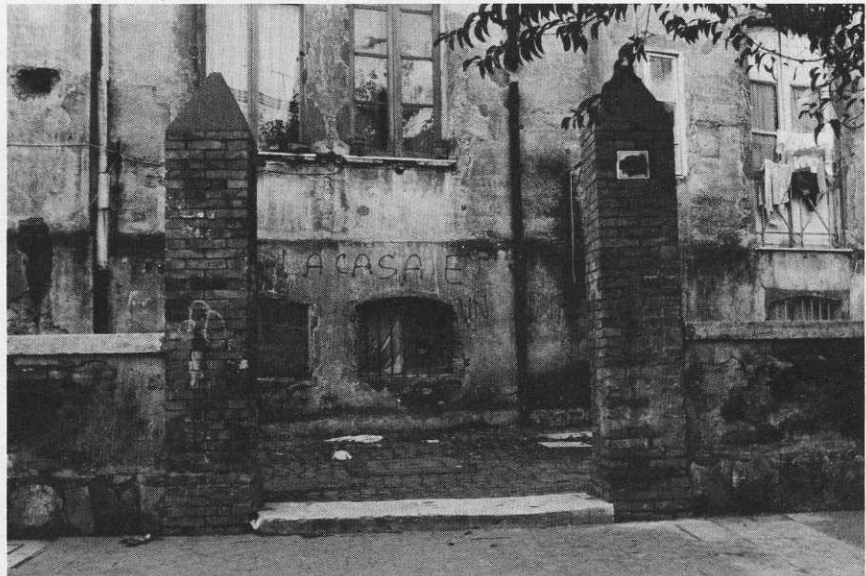
Lucas's headquarters at the beginning of February was located in the old Italian artillery barracks at No. 39 Via Santa Maria. Today the building is in poor shape presenting a very run-down appearance much out of keeping with its historic past.
